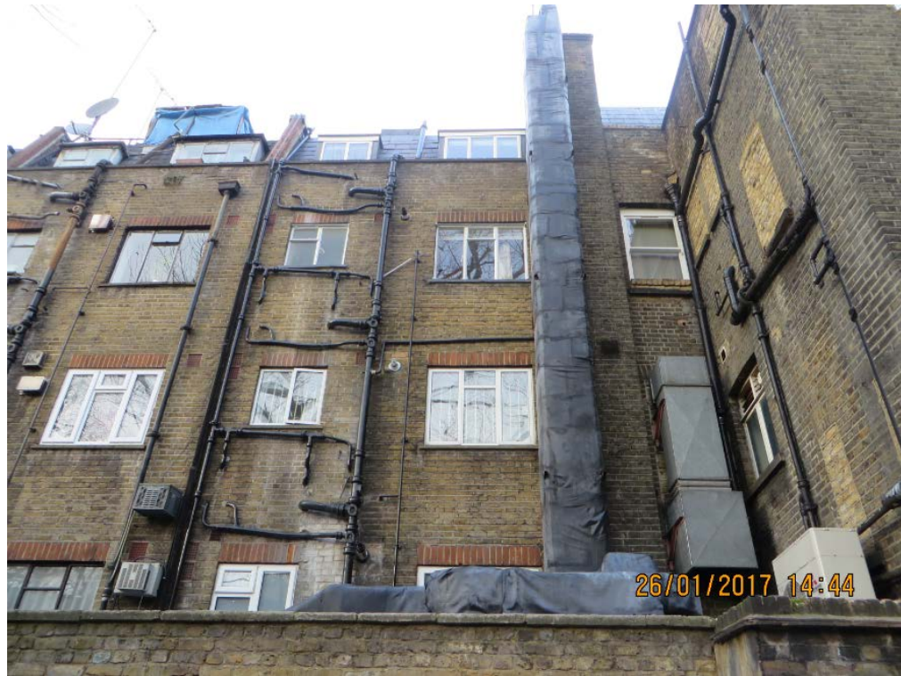
Unauthorised extract duct
