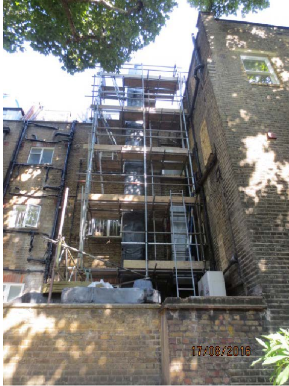
Unauthorised extract duct
